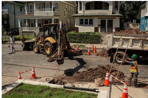
Workers removing lead pipes in Newark, N.J. $45 billion goes toward elimination of lead pipes. Credit - Bryan Anselm for The New York Times
